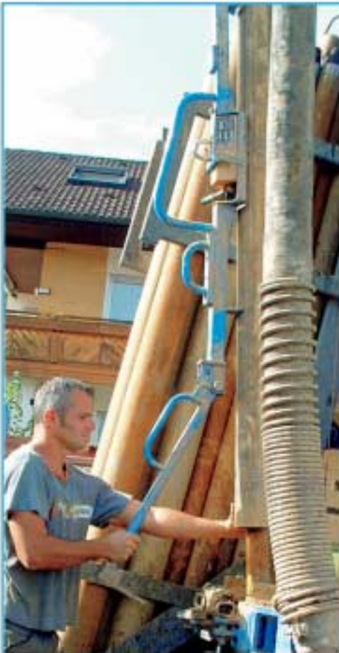
Handling system with magnet for casing and rods.
